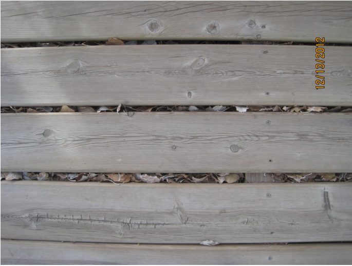
Leaf and litter buildup in decks and porches.
