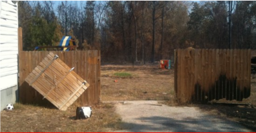
The attached wooden fence almost got this house burned down. Firefighters opened the gate to keep the fence fire away from the house.
