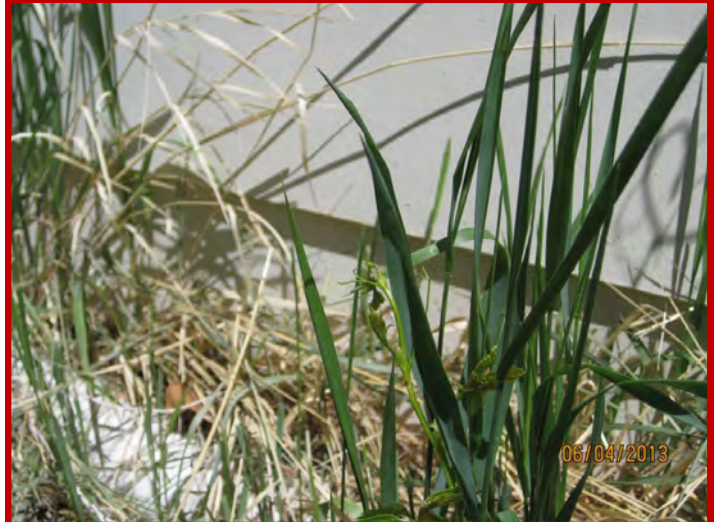
Cured grass in contact with an outside wall
