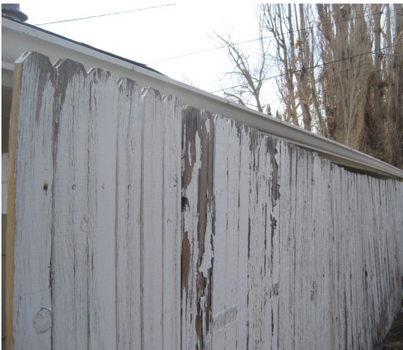
A weathered fence under the eaves—not good.
