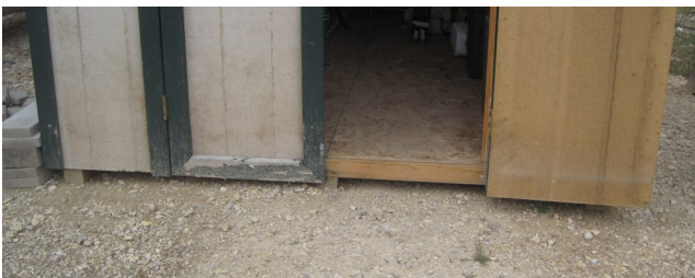
Gravel and sand under & around storage shed
