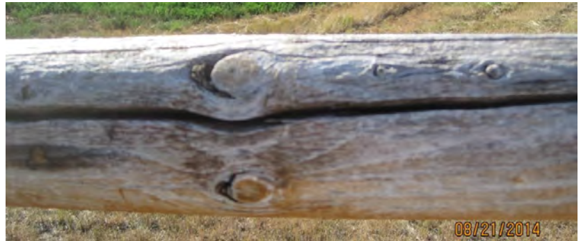
This wide crack in a old and dried porch railing is an ember trap.
