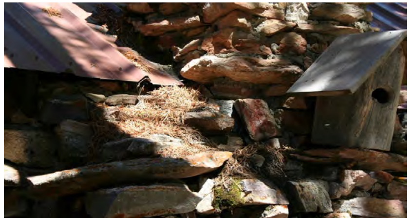
Flammable tree needles under the eaves by a chimney.
