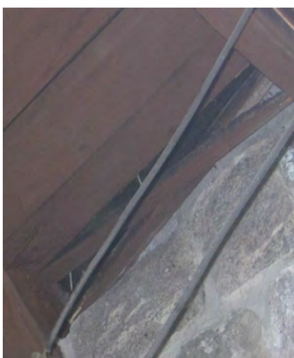
Broken under-eave boards would allow entry of embers
