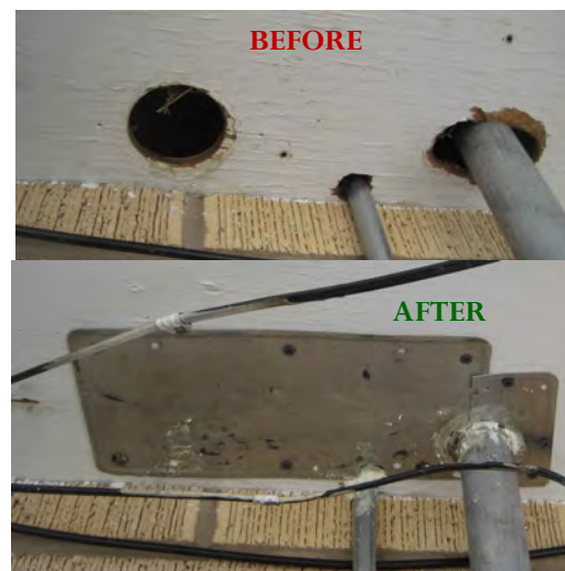
Eave openings permanently covered with thin metal (a license plate), with sealed seams
