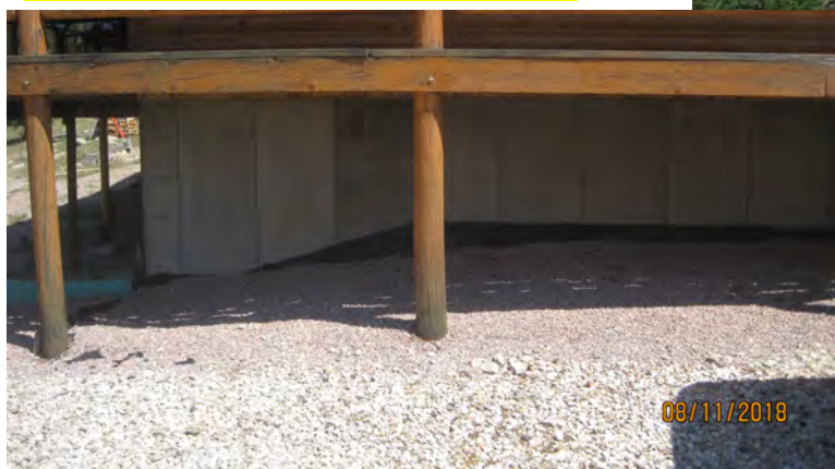
An under-deck area kept free of flammable materials, and surfaced with gravel to protect the foundation from fire.
