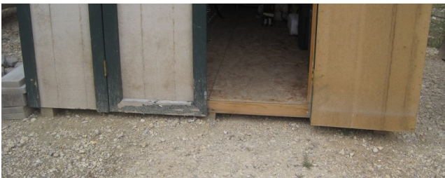
Gravel and sand under & around storage shed
