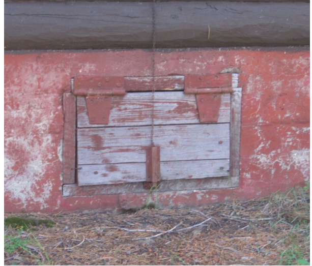
Exposed uncoated access hatch
